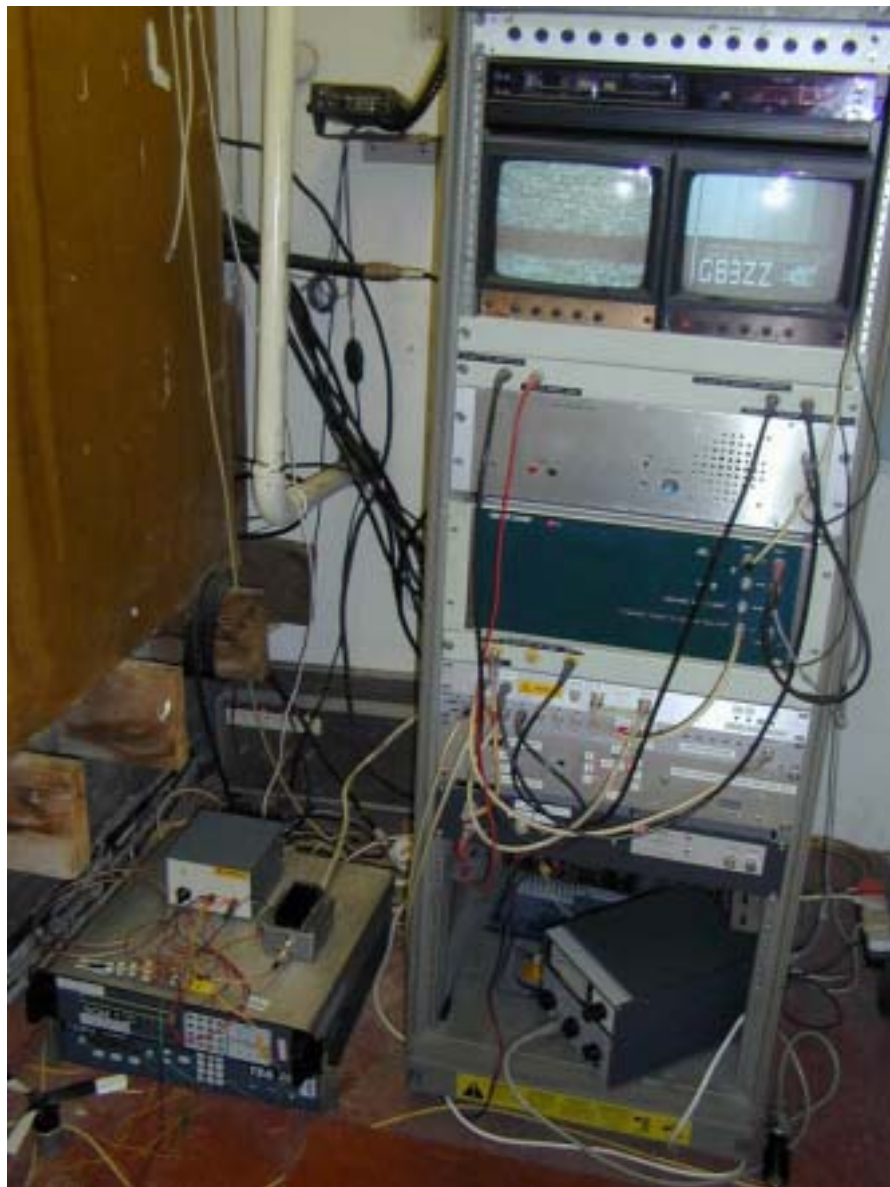
Transmit equipment in shack with GB3ZZ
